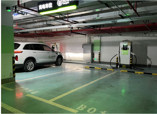
Nantong Innovation Center Station-30KW charging module
