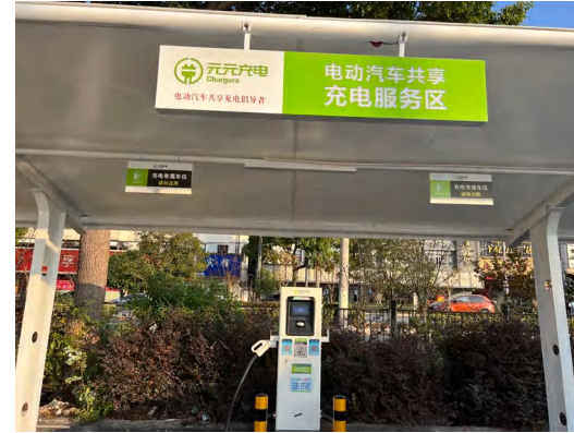
Hotel Station - 30KW charging module
