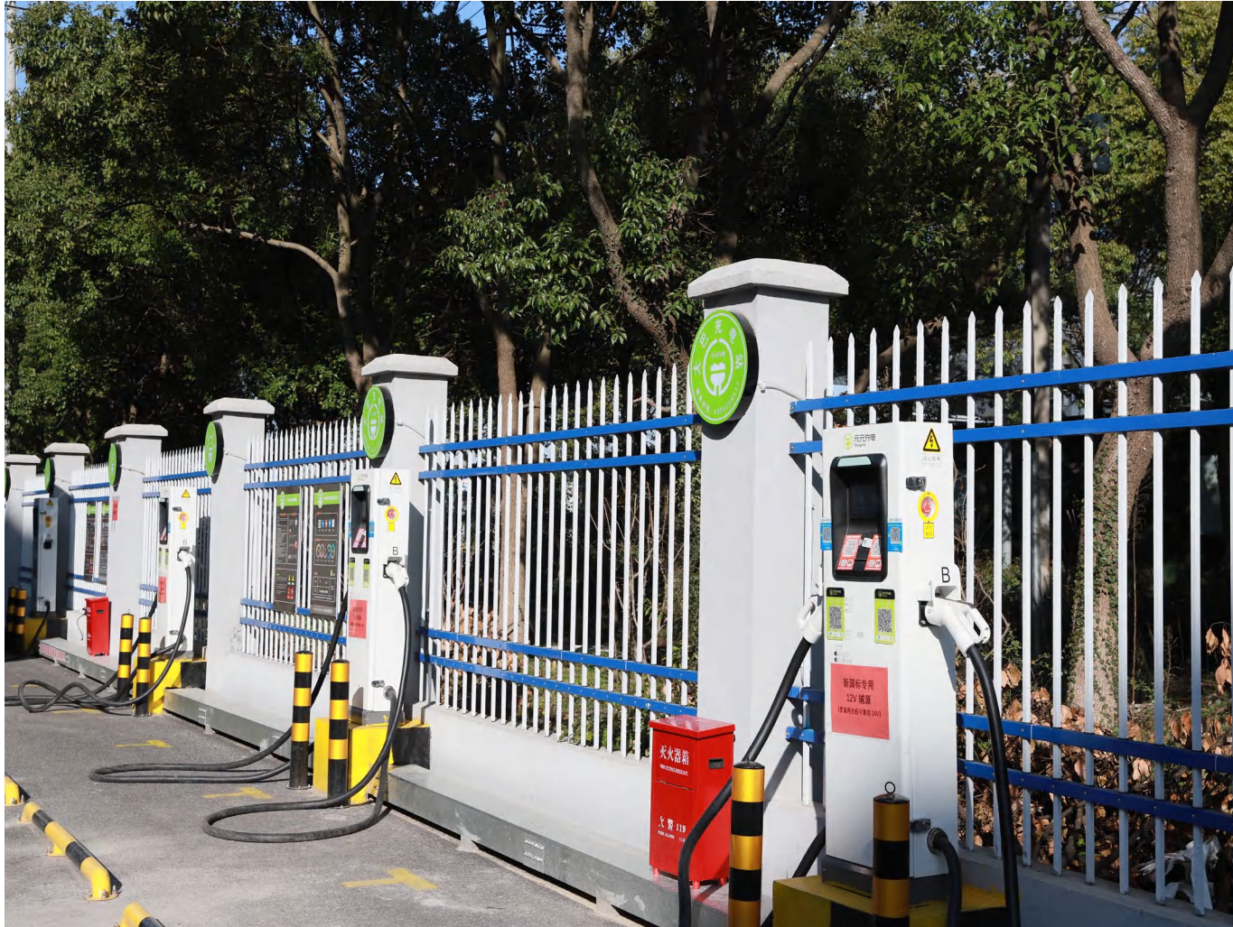
E-Bus Charging Station - 30KW charging module
