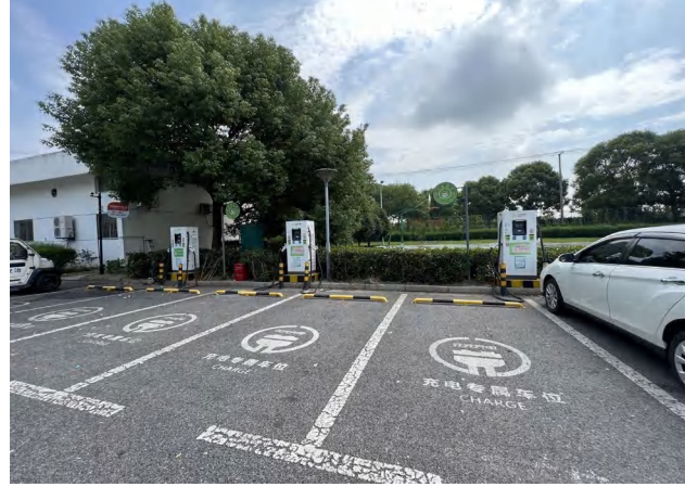
Comprehensive Bonded Zone Station-20KW Charging Module
