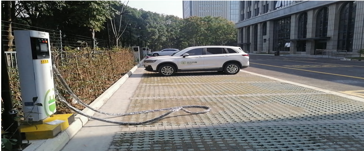
Taigu Plaza Station-30KW charging module (silicon carbide)
