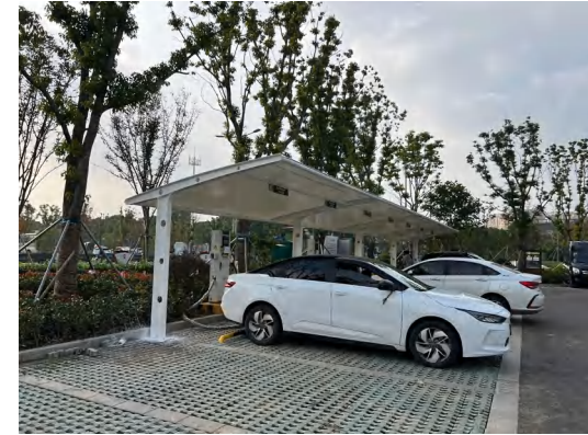
XinHuangDai Charging Station -30KW charging module
